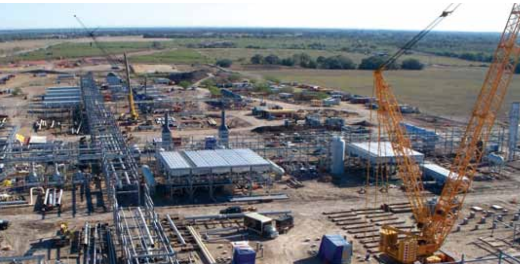
KCTG's Optimized Process Designs was chosen to design and build this plant for processing gas liquids from Eagle Ford.
